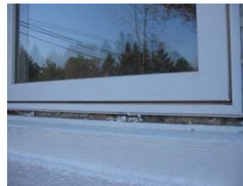
"Many windows are in poor condition"
