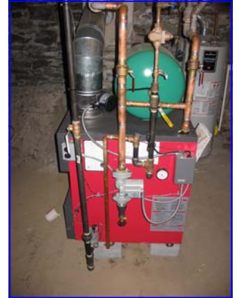
"Old furnaces and boiler are very inefficient compared to newer models"
